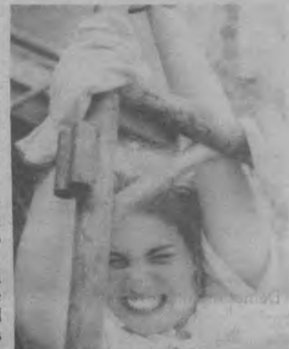
Joanna Weiner puts all her energy into the building of the scaffolding at the beginning of a day's work at Delamore Place. (Photo: Jonathan Hirsch)
