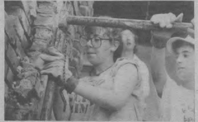
Eden Feirstein and Dan Weiner work at removing a steel railing from the brick wall at the Delamore Place address which is their summer renovation site. (Photo: Jonathan Hirsch)
