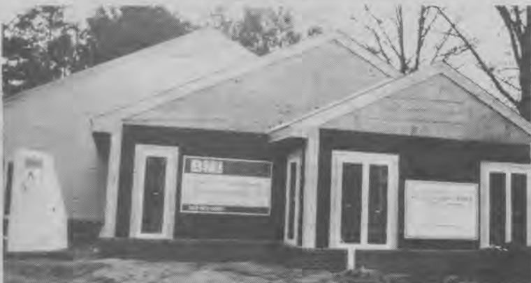
The Abe and Pearl Kristol Hillel Student Center at the University of Delaware currently under construction is scheduled to open February 1993.
