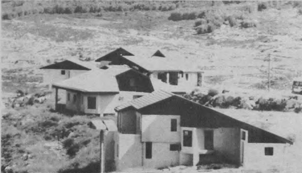
BUILDING FOR TOURISM IN ISRAEL'S GALILEE. New construction, such as that shown above, is underway in Israel's Galilee, its northern section, where tourism is expected to become an increasingly important industry. American Jews are playing a role in development here through the UJA/Federation Campaign. — UJA Press Service Photo
