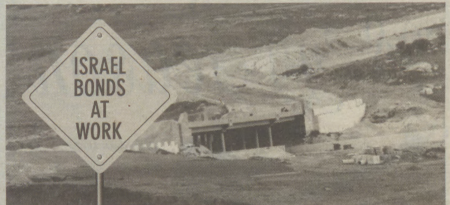
The Bet Shemesh Bridge, under construction in 1998, links the old city to the rapidly growing new city.
