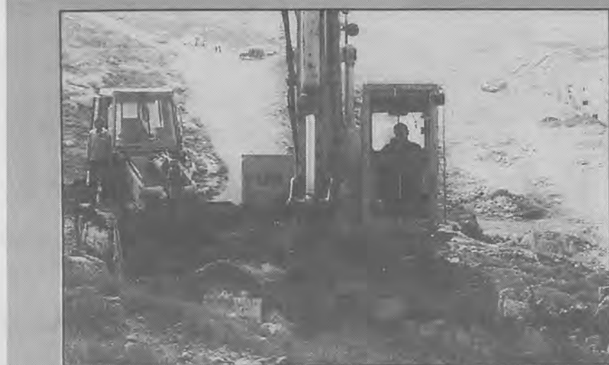
AL-KHADER, West Bank -- Bulldozers break ground for new settler homes above Efrat settlement Jan. 4, near where Israeli troops and Palestinian protesters clashed recently over plans to build on what Arab villagers claim is their land. The Israeli government, under pressure from Palestinians, halted work on the disputed hill near al-Khader village, but authorized work on the land closer to Efrat. At press time the Government hinted at strong support for Israeli development within Jerusalem borders. CREDIT:RNS PHOTO/Reuters (Reproduction rights not transferable)
